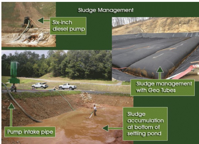
Figure 16. Conventional Acid Mine Drainage Sludge Treatment.
